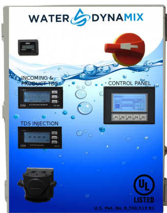
Water Dynamix—Control Panel
